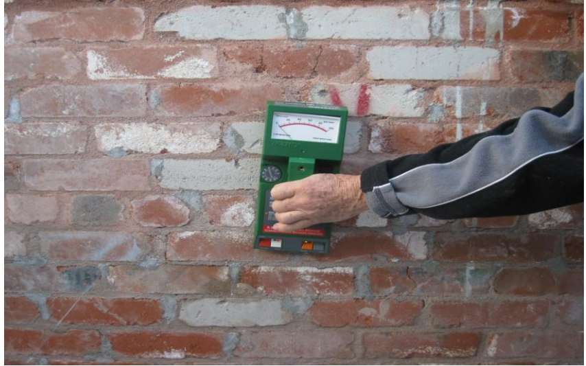
Figure 6. Moisture meter in use on a clay masonry wall. Values indicated by meter are relative moisture content based on calibration with each particular material.
