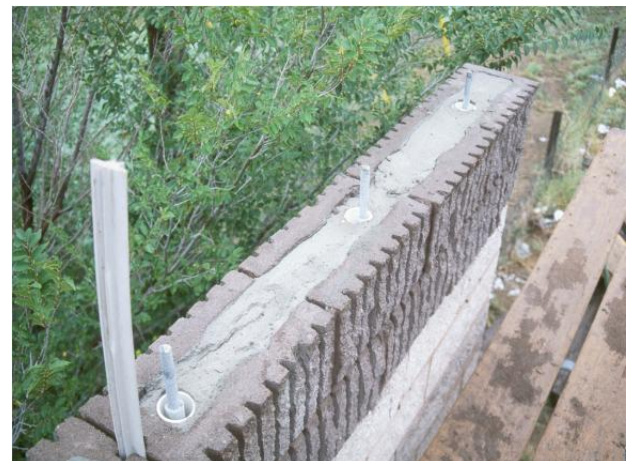
Bond beam and tendons at top of post-tensioned wall.
