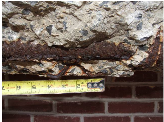
Close-up view of steel reinforcing with corrosion
