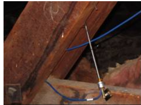
Gauge for monitoring truss movement
