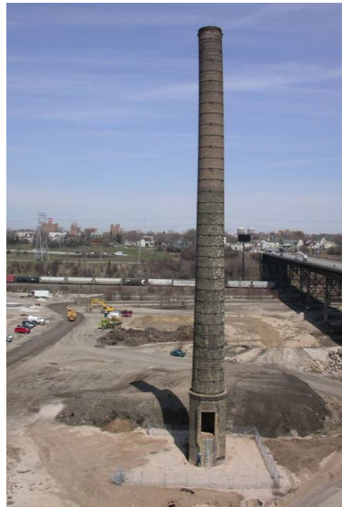
A 100 ft. lift was used to access the lower portion of the 200 ft tall stacks.
