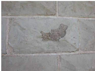
Typical delamination in site-cast units
