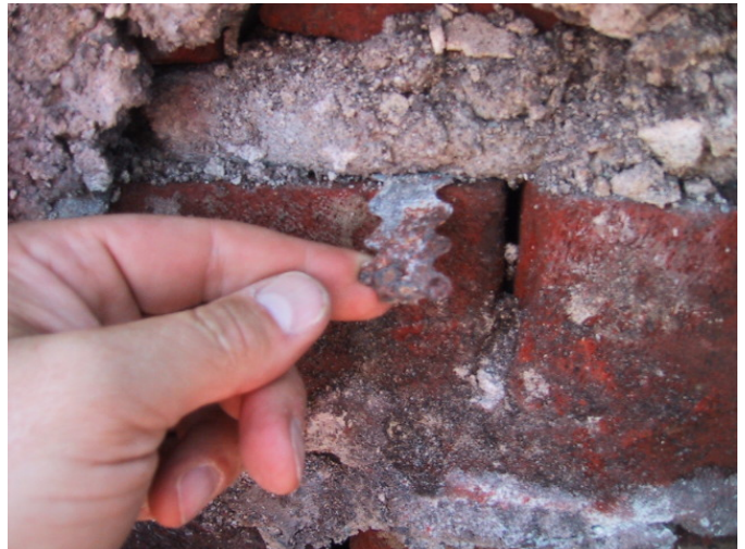
Corroded metal wall tie
