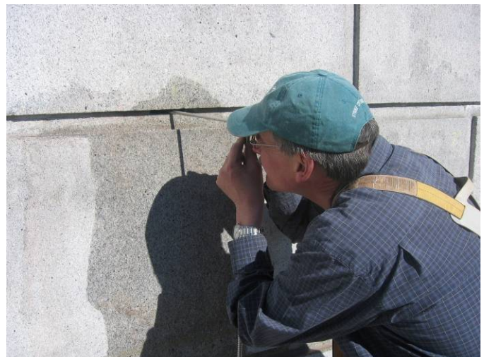
Use of borescope to investigate wall construction and condition of metal ties
