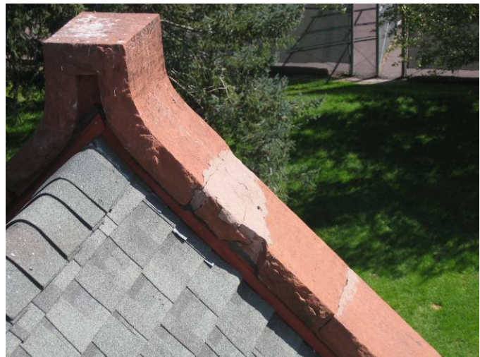
Stone deterioration at roof
