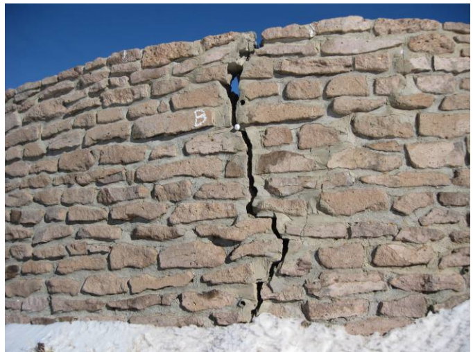
Typical wall crack at the Cedar Breaks Overlooks
