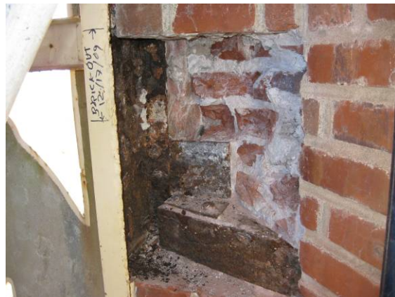
Typical corrosion damage of steel elements at the Bok Tower.
