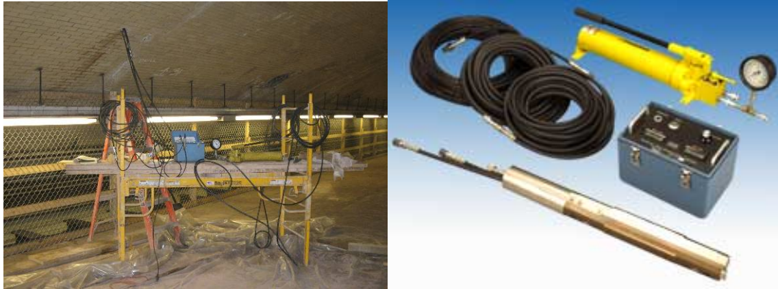
Goodman jack testing to measure the stiffness of the masonry at various depths within a 4-inch core hole (photograph on right courtesy of Durham Geo Slope Indicator).
