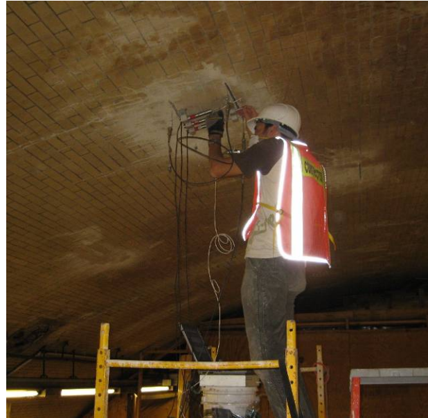
ANA Engineer conducting flatjack test to determine compressive deformability of the brick masonry vault.
