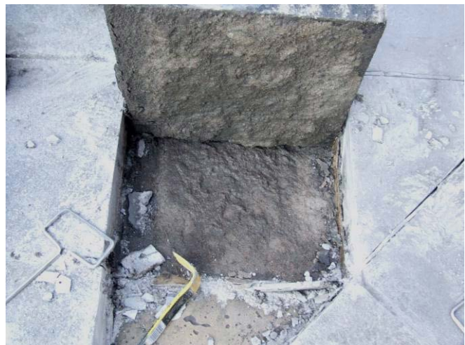
View of a granite paver being removed as part of maintenance operations.
